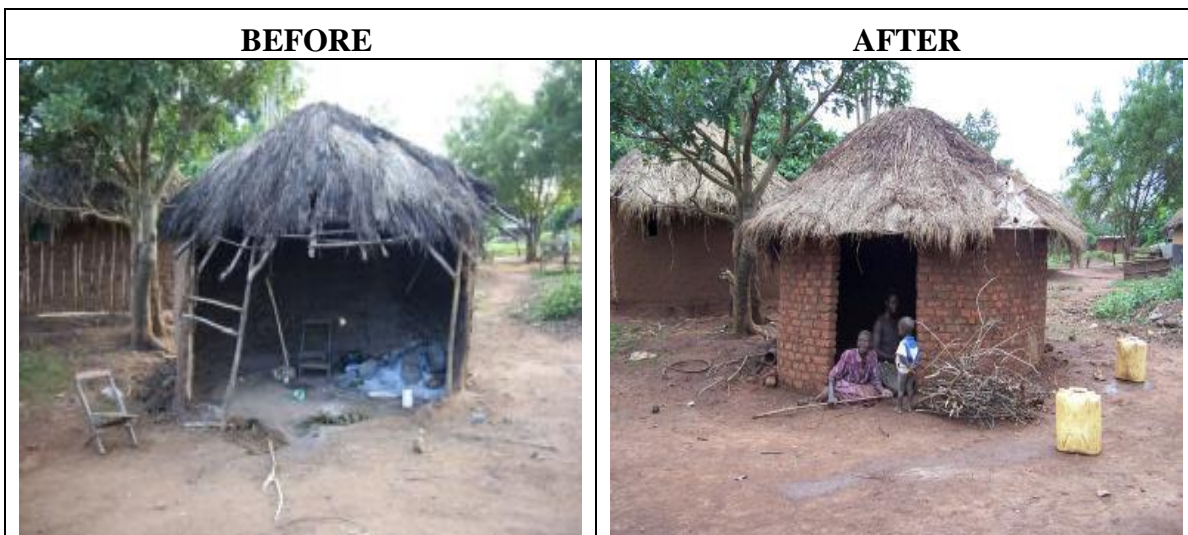
Fig. 3 – An open and dilapidated kitchen is exposed to rain and disease spreading vectors such as rats. In securing the structure and entrance we reduce the risk and allow for cooking during rainy seasons.
